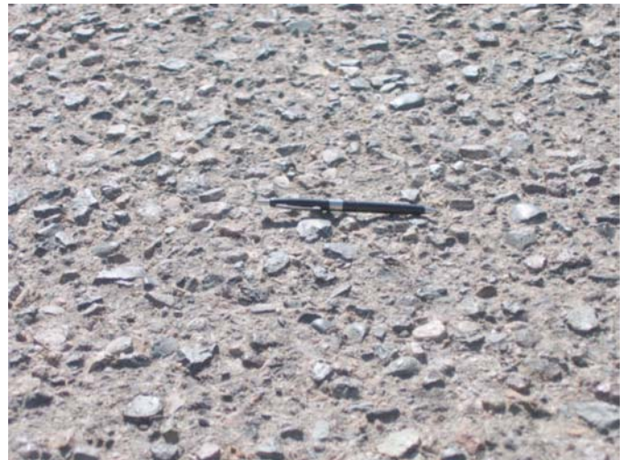
FIG. X1.55 High-Severity Weathering (Surface Wear)
