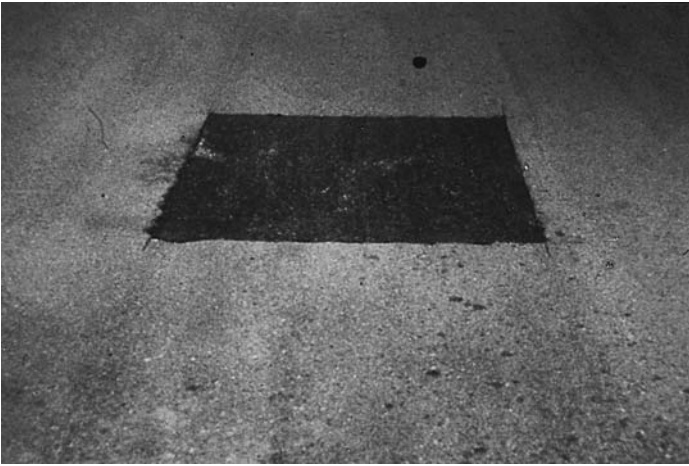
FIG. X1.31 Low-Severity Patching and Utility Cut Patching
