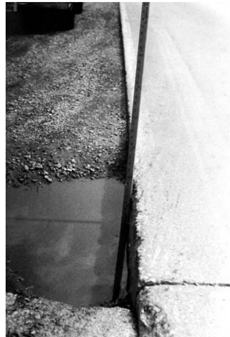
FIG. X2.21 High-Severity Lane/Shoulder Drop-Off
