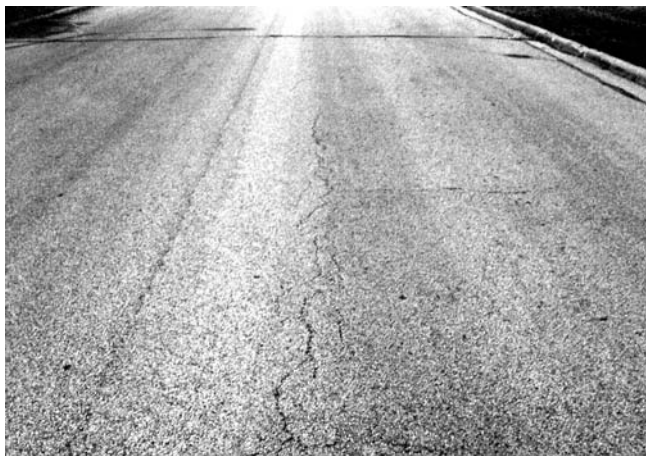
FIG. X1.1 Low-Severity Alligator Cracking
