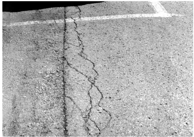
FIG. X1.20 Medium-Severity Edge Cracking
