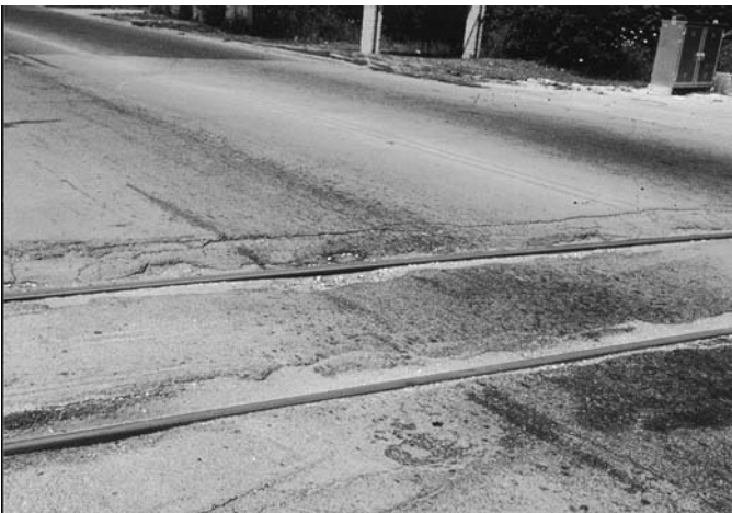
FIG. X1.39 Medium-Severity Railroad Crossing
