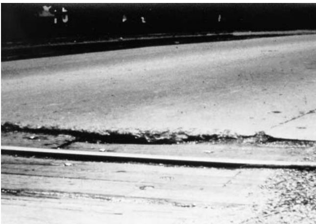
FIG. X2.40 High-Severity Railroad Crossing
