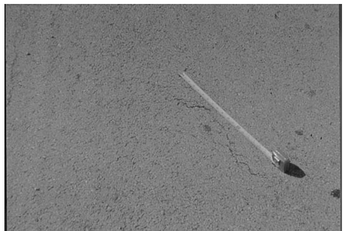
FIG. X1.47 Low-Severity Slippage Cracking
