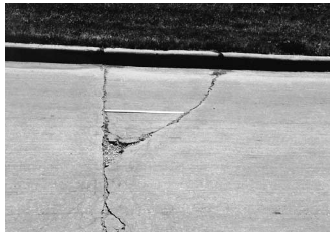
FIG. X2.5 Medium-Severity Corner Break
