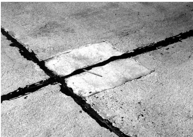
FIG. X2.28 Low-Severity Patching, Small
