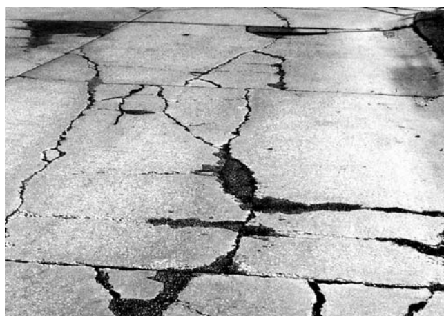
FIG. X2.9 High-Severity Divided Slab
