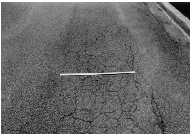
FIG. X1.2 Medium-Severity Alligator Cracking
