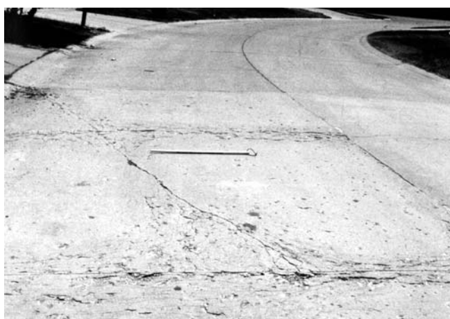
FIG. X2.12 High-Severity Durability Cracking
