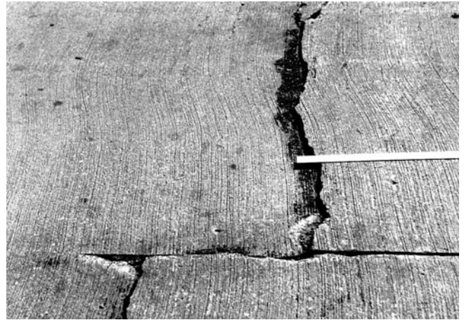
FIG. X2.24 High-Severity Linear Cracking
