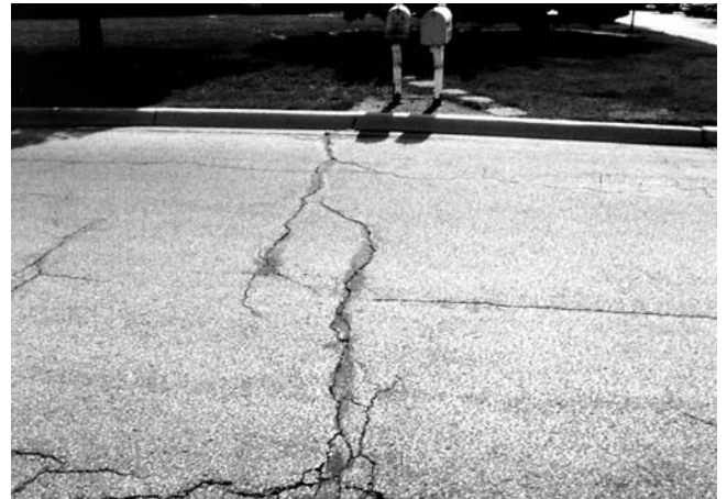
FIG. X1.8 Medium-Severity Block Cracking
