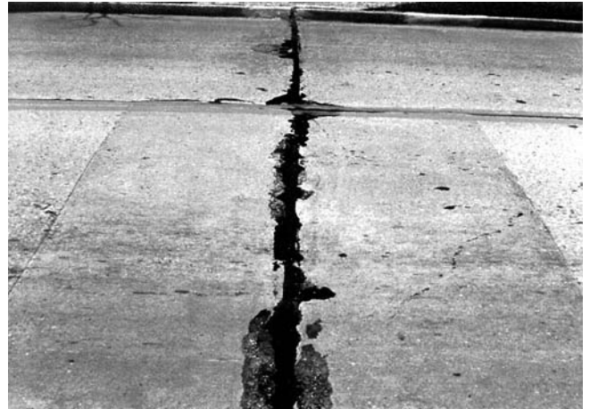
FIG. X2.16 Low-Severity Joint Seal Damage
