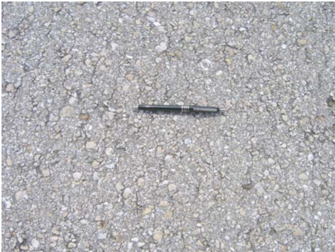
FIG. X1.53 Low-Severity Weathering (Surface Wear)
