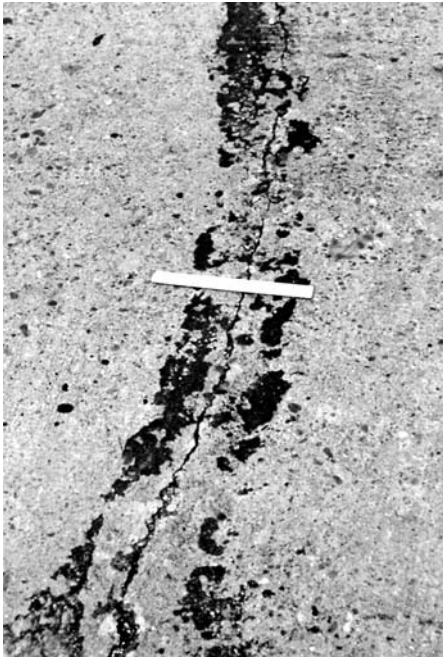
FIG. X2.22 Low-Severity Linear Cracking
