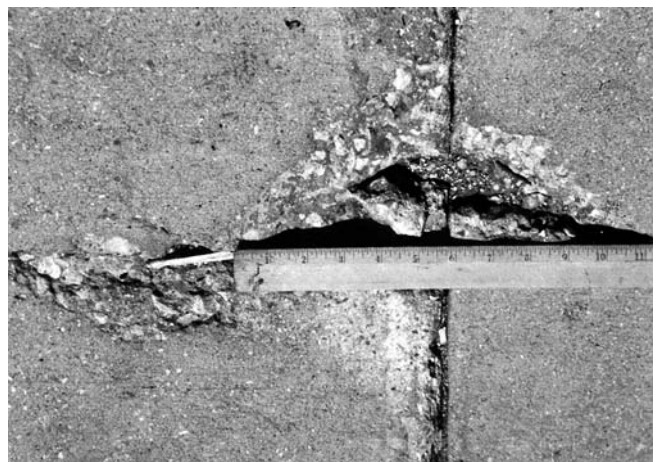
FIG. X2.46 Medium-Severity Spalling, Corner
