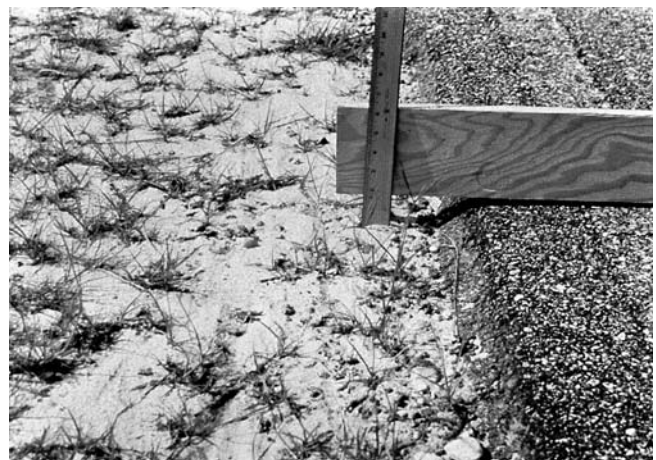
FIG. X1.25 Low-Severity Lane/Shoulder Drop-Off
