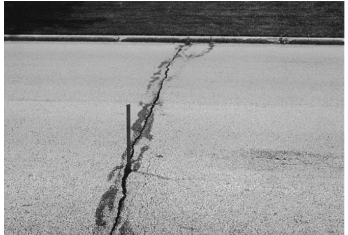
FIG. X1.29 Medium-Severity Longitudinal and Transverse Cracking
