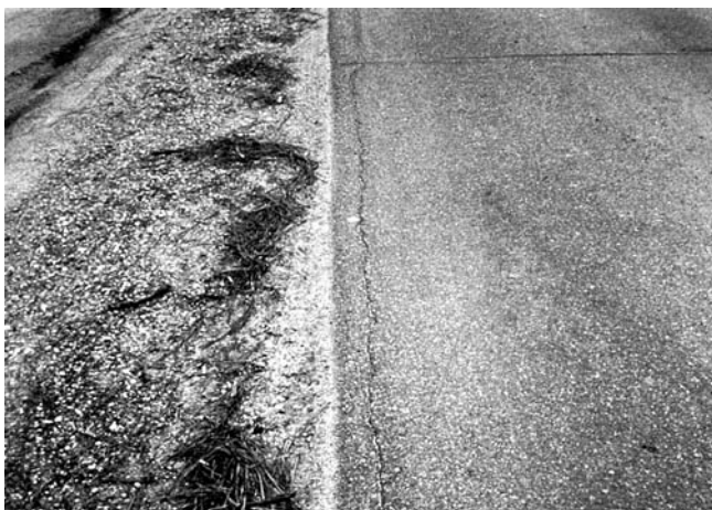
FIG. X1.19 Low-Severity Edge Cracking
