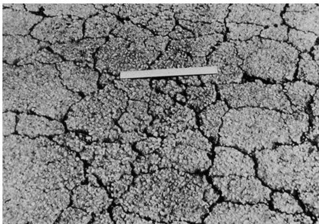
FIG. X1.3 High-Severity Alligator Cracking
