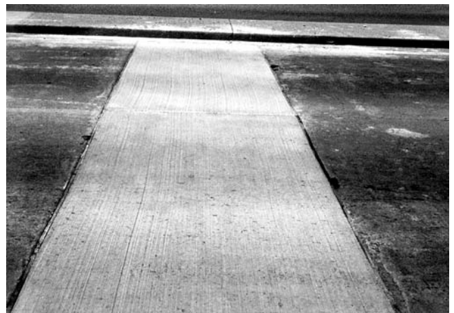
FIG. X2.25 Low-Severity Patching, Large and Utility Cuts
