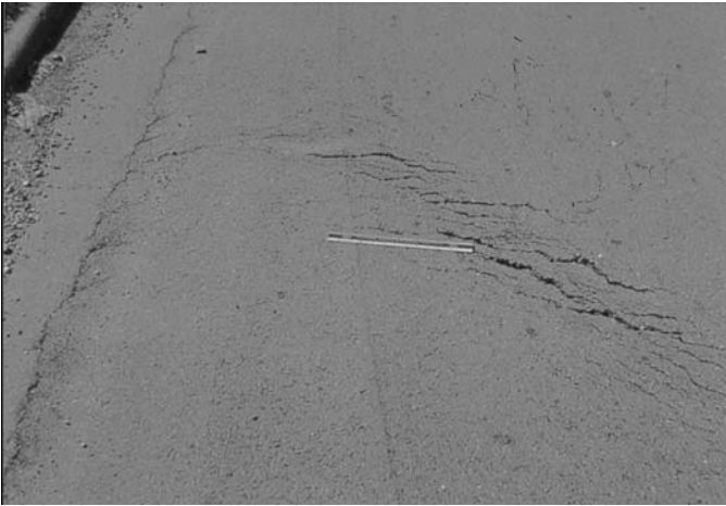
FIG. X1.48 Medium-Severity Slippage Cracking
