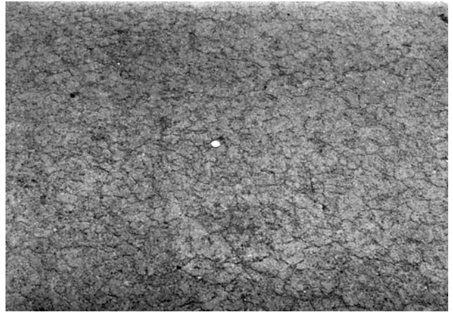
FIG. X2.41 Low-Severity Scaling, Map Cracking, and Cracking
