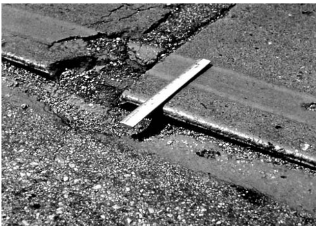
FIG. X2.19 Low-Severity Lane/Shoulder Drop-Off
