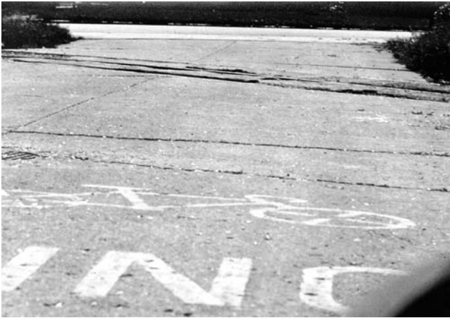
FIG. X2.39 Medium-Severity Railroad Crossing
