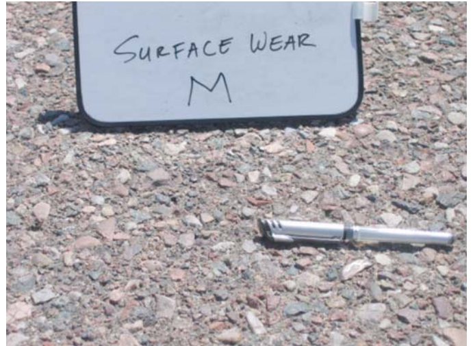
FIG. X1.54 Medium-Severity Weathering (Surface Wear)
