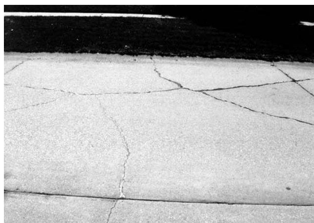
FIG. X2.8 Medium-Severity Divided Slab
