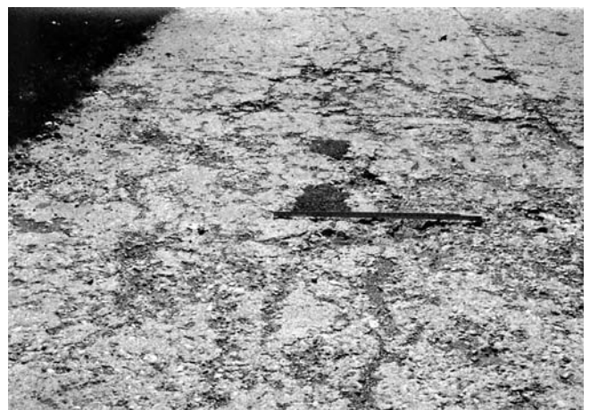
FIG. X2.43 High-Severity Scaling, Map Cracking, and Cracking
