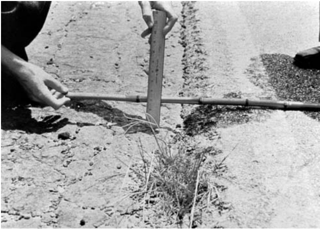
FIG. X1.26 Medium-Severity Lane/Shoulder Drop-Off
