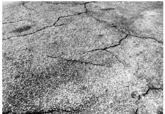
FIG. X1.9 High-Severity Block Cracking
