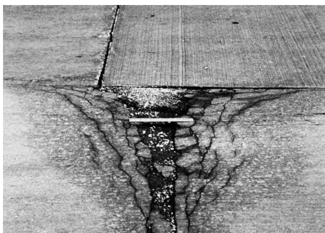
FIG. X2.11 Medium-Severity Durability Cracking
