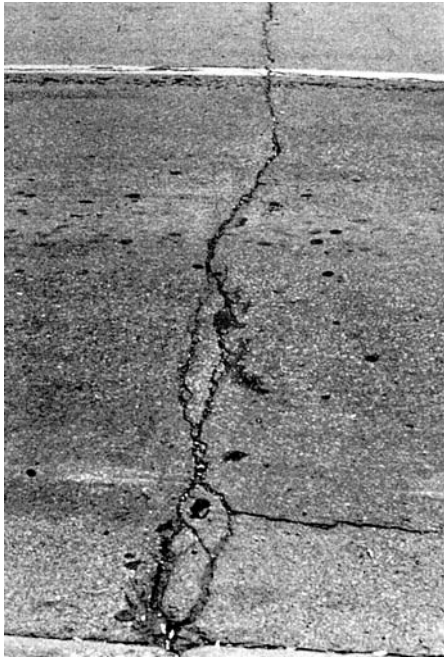
FIG. X1.23 Medium-Severity Joint Reflection Cracking
