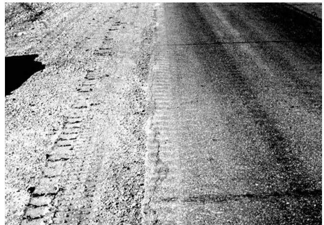
FIG. X1.22 Low-Severity Joint Reflection Cracking
