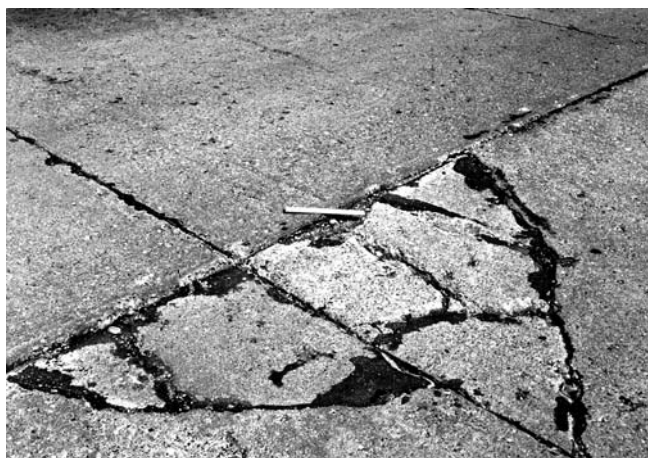
FIG. X2.6 High-Severity Corner Break
