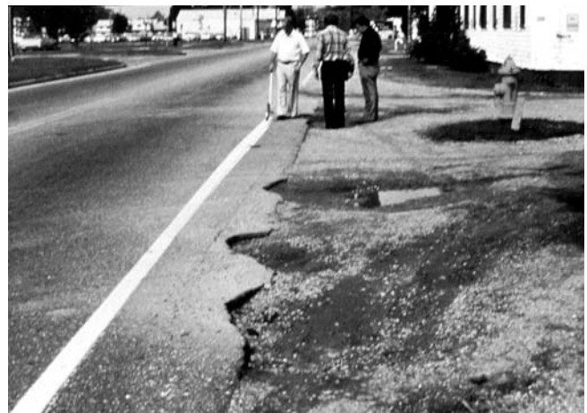
FIG. X1.21 High-Severity Edge Cracking
