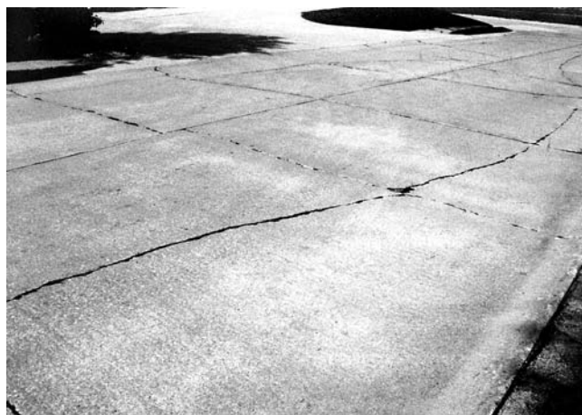
FIG. X2.7 Low-Severity Divided Slab
