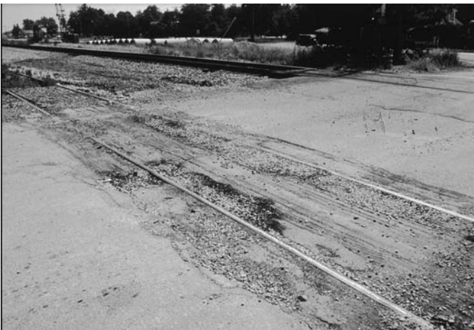
FIG. X1.40 High-Severity Railroad Crossing
