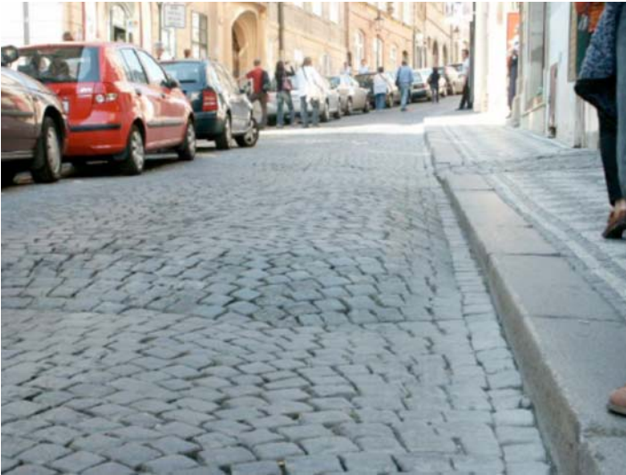
FIG. X1.18 High Severity Heave
