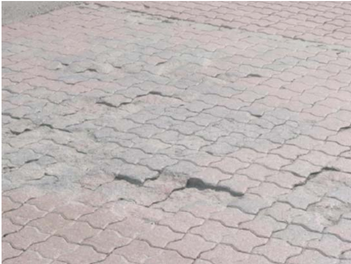
FIG. X1.3 High Severity Damaged Pavers
