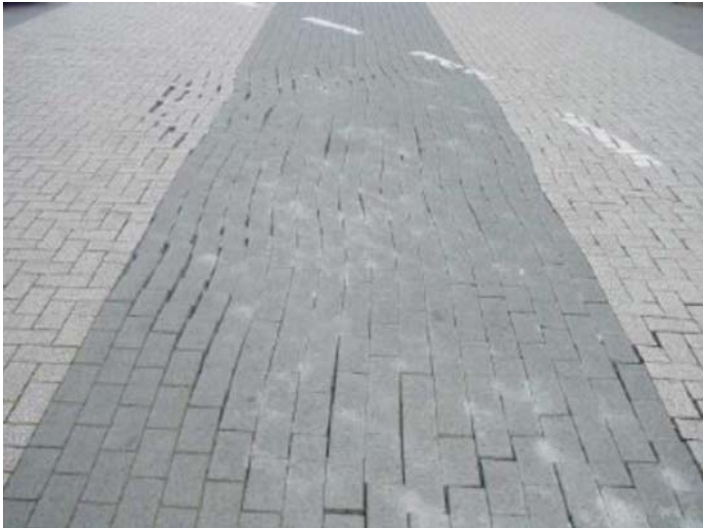
FIG. X1.9 High Severity Loss of Edge Restraint
