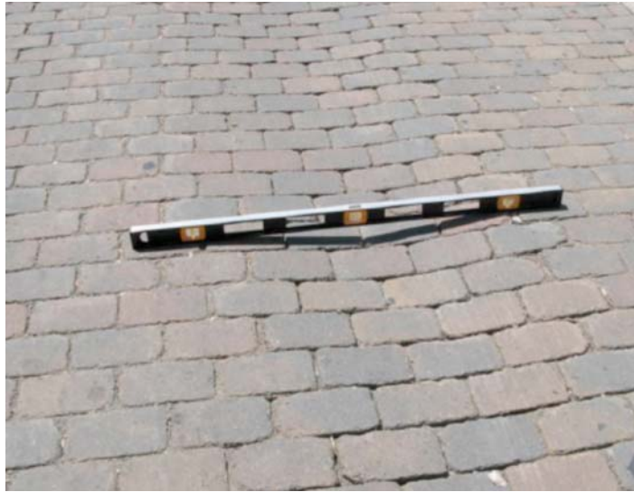
FIG. X1.33 High Severity Rutting
