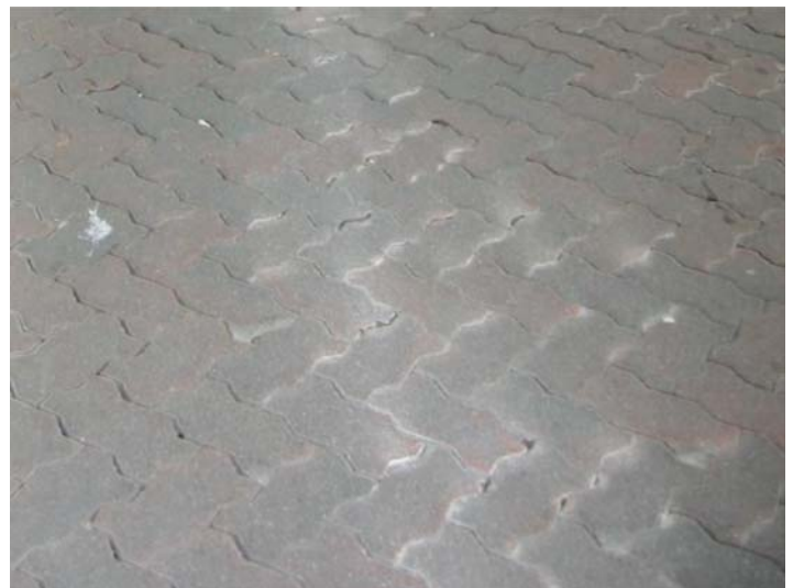
FIG. X1.23 Medium Severity Joint Sand Loss
