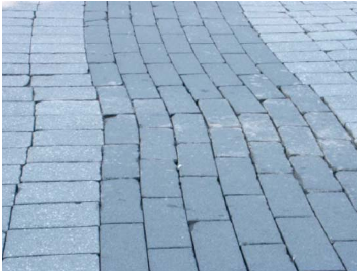
FIG. X1.21 High Severity Horizontal Creep
