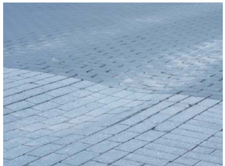
FIG. X1.32 Medium Severity Rutting
