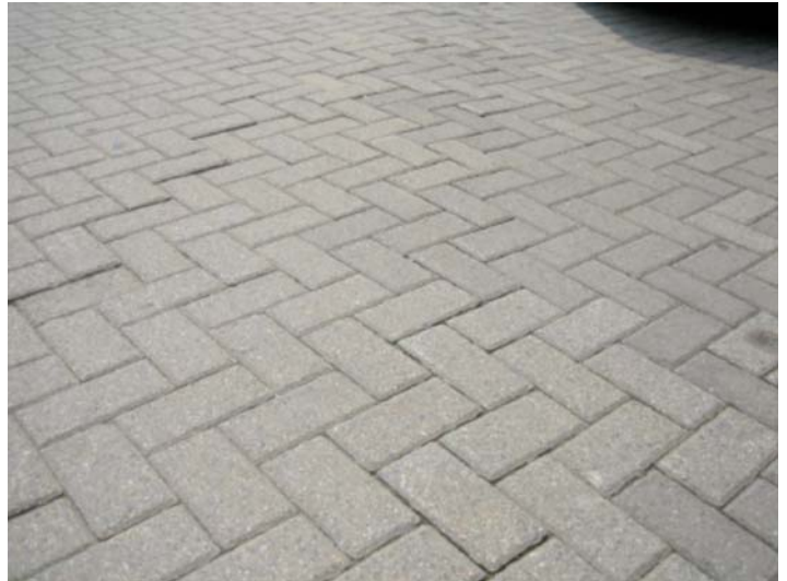
FIG. X1.13 Low Severity Faulting
