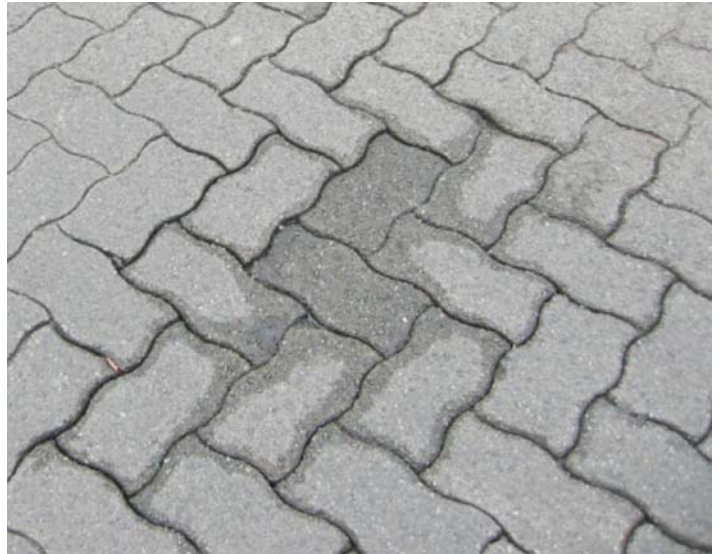
FIG. X1.10 Low Severity Excessive Joint Width (Approximately 1/4 in. (6 mm) wide and performing well)
