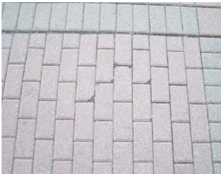
FIG. X1.1 Low Severity Damaged Pavers
