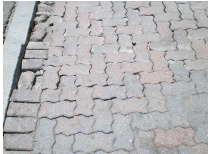
FIG. X1.8 Medium Severity Loss of Edge Restraint
