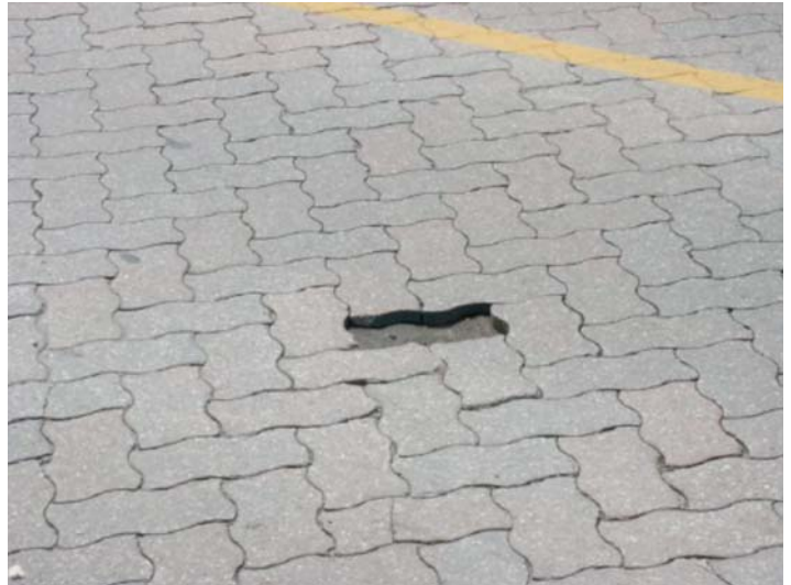
FIG. X1.25 Low Severity Missing Pavers
