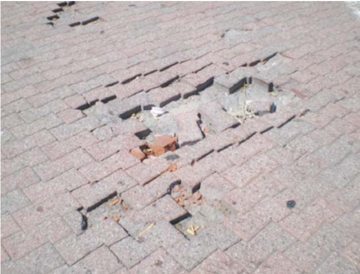
FIG. X1.27 High Severity Missing Pavers
