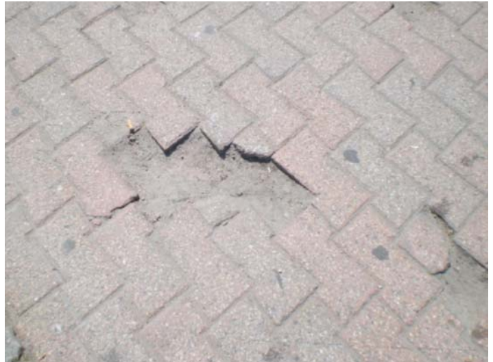
FIG. X1.26 Medium Severity Missing Pavers
