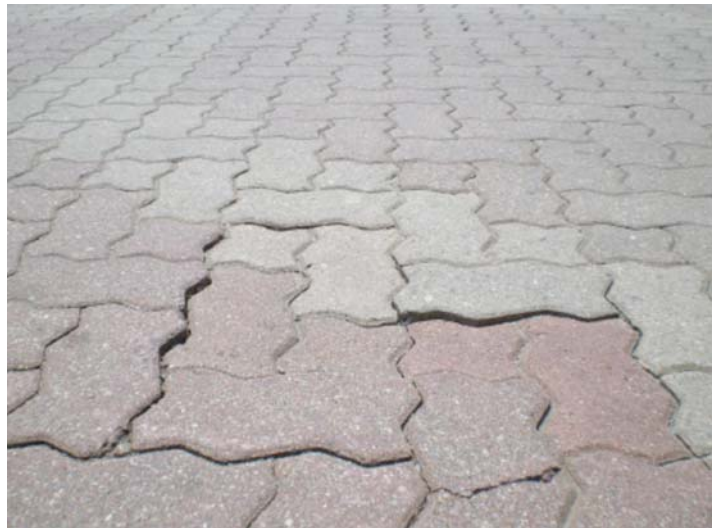
FIG. X1.14 Medium Severity Faulting
