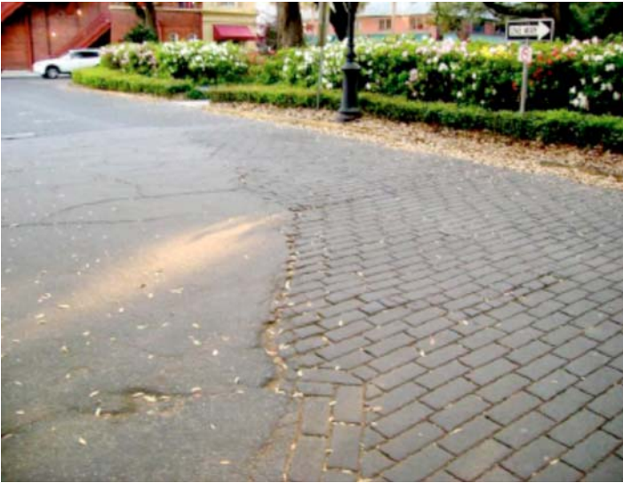
FIG. X1.29 Medium Severity Patch
