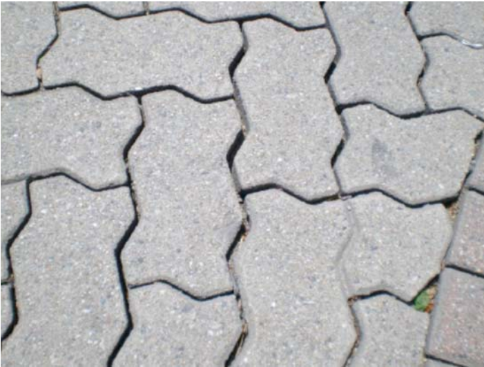
FIG. X1.24 High Severity Joint Sand Loss
