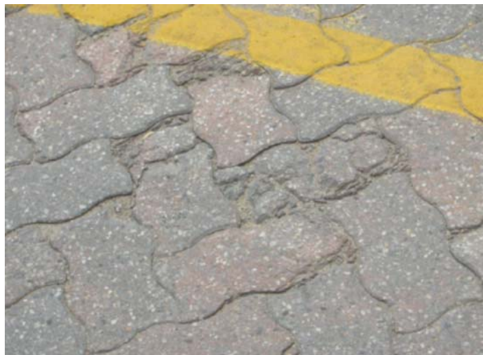
FIG. X1.2 Medium Severity Damaged Pavers
