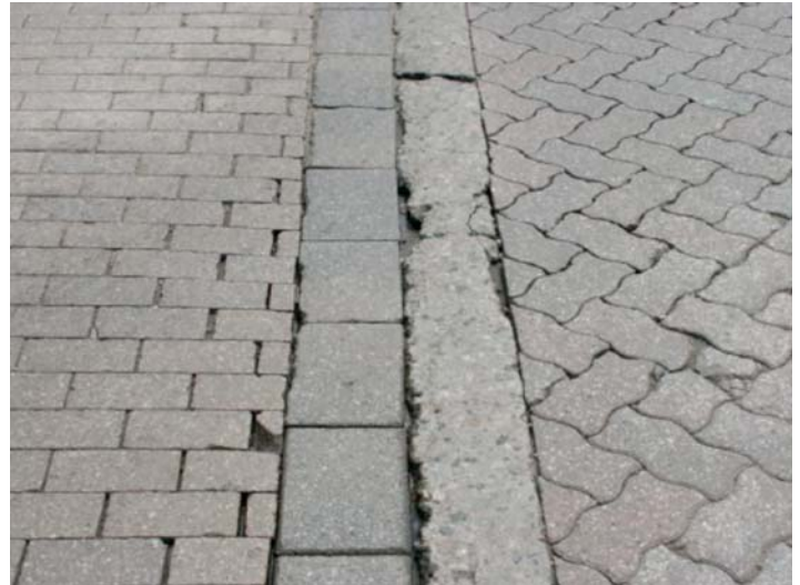
FIG. X1.7 Low Severity Loss of Edge Restraint
