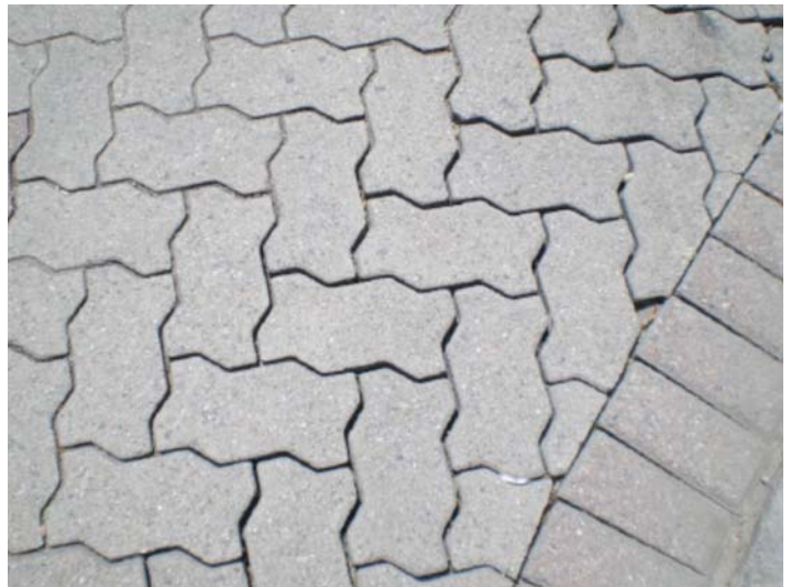
FIG. X1.11 Medium Severity Excessive Joint Width
