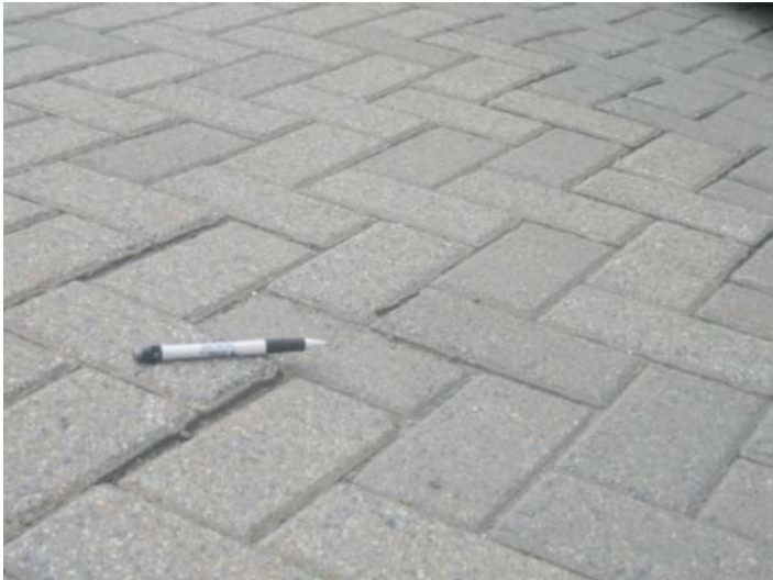
FIG. X1.15 High Severity Faulting
