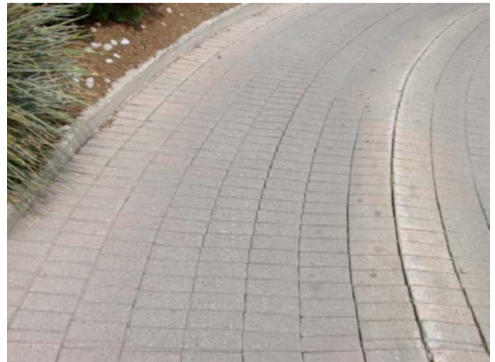
FIG. X1.31 Low Severity Rutting
