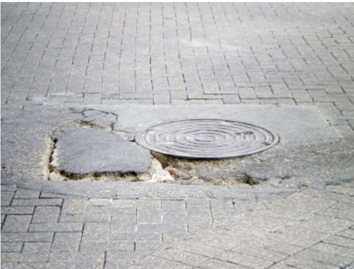
FIG. X1.30 High Severity Patch
