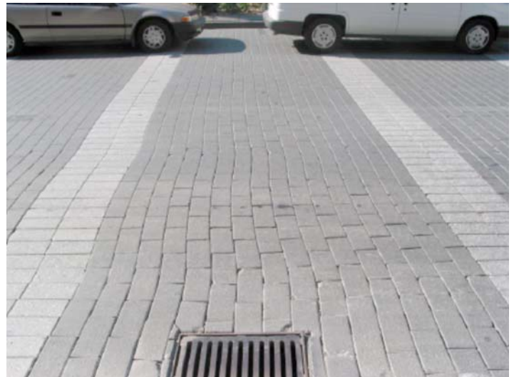
FIG. X1.20 Medium Severity Horizontal Creep
